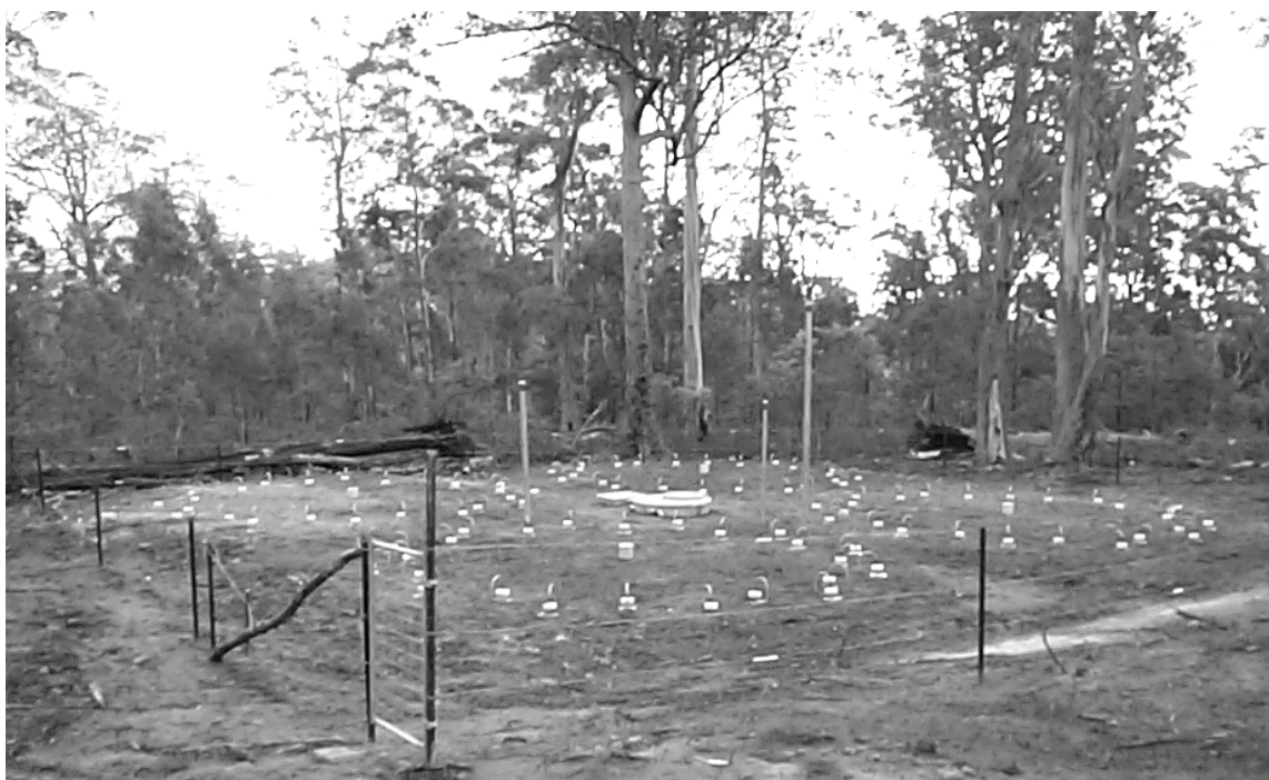
Figure 3—The Buckland Infrasound Station was constructed during 2002-2003 at the Buckland Military Training Area in central Tasmania. Photo courtesy of Geoscience Australia.
