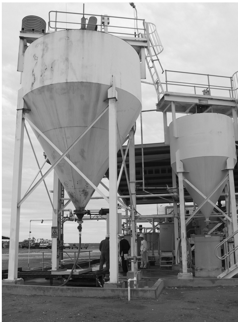
Figure 5—Uranium ore container filling facility, Honeymoon uranium mine.
